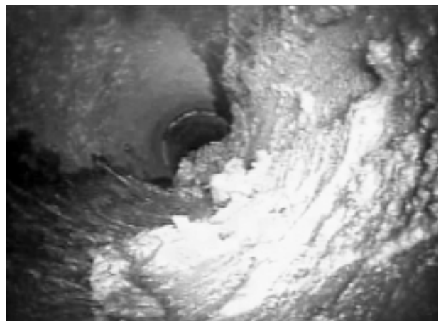
SeeSnake picture of semi collapsed pipe.
