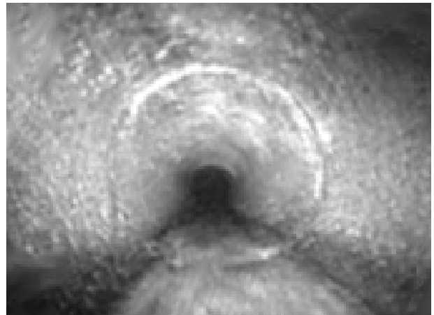
SeeSnake picture of line with no defects.
